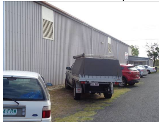
The new vents from the outside .....
